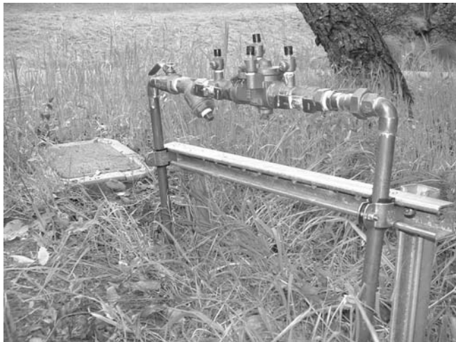
Installed reverse pressure zone device
